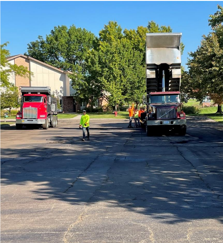
Workmen from McKearney Asphalt prepare to resurface The PCO parking lot in the fall of 2021.
